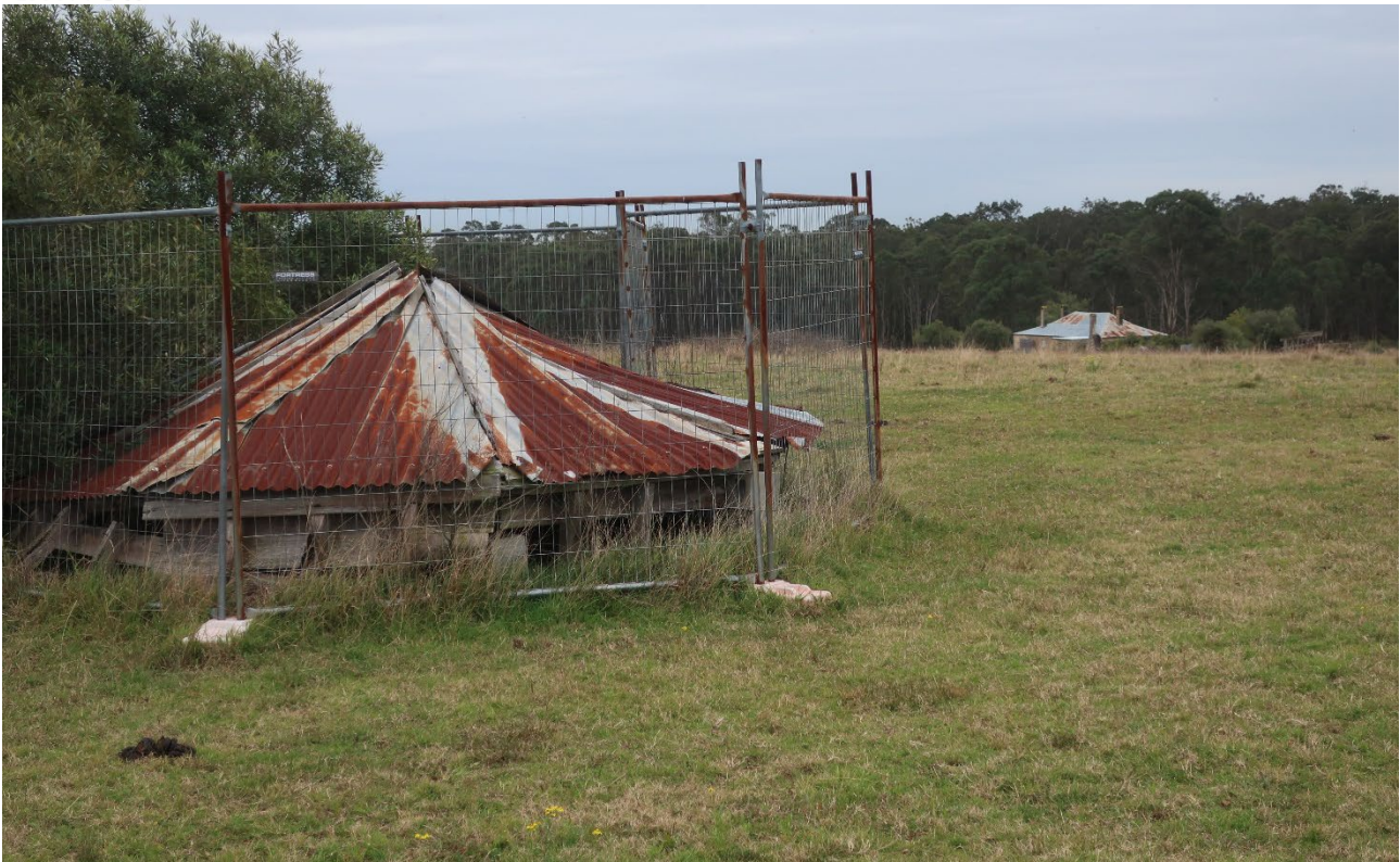
Photo 4-4 The collapsed gazebo of Beulah is close to the boundary with Meadowvale
